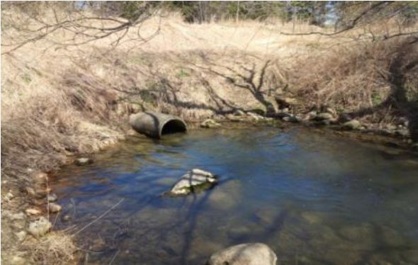
A 762 mm diameter (inner) concrete pipe conveys flow from the pond to a pool at the creek outlet.
