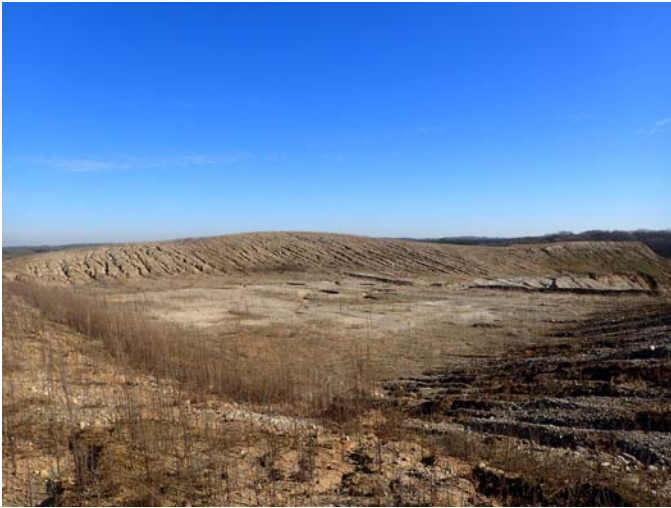
2020/11/09 13:44:38 TG-4;PB090110.JPEG Taken by: Stephen Douglas View E toward the N end of the Interim Berm which has been graded and seeded
