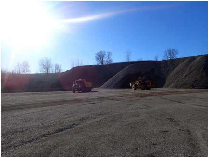
2020/11/09 14:16:31 TG-4;PB090118.JPEG Taken by: Stephen Douglas Loading of a dump truck in the S part of Area 1
